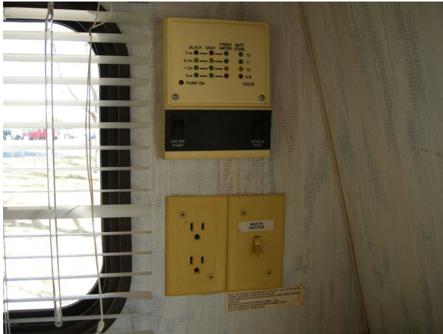
Photo of trailer control panel located on street side forward of the stove.
