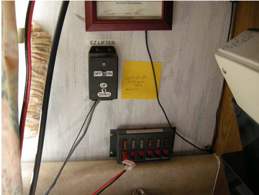
Photos of Power antenna and control switch, located just aft of window in radio room on curb side of trailer.
